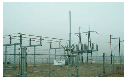
▲ Figure 13-7 Part of the electrical transmission network in Alberta, near Lethbridge. The Alberta government is reviewing its restructuring of the electrical energy industry. It has set 2012 as the new target date for achieving a competitive free market for electricity. However, there is some concern over the impact of the Kyoto Protocol if generation plants have to meet the Protocol's environmental standards. How might the government see the Kyoto Protocol as both an opportunity and a challenge?
